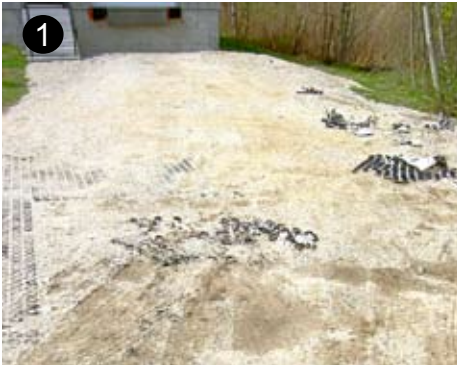
Failed Gravelpave2 Installed System
